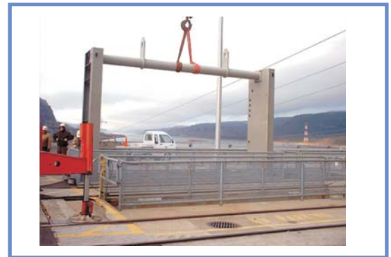
Lowering ASFM frame at U.S. Army Corps of Engineers' John Day dam site
